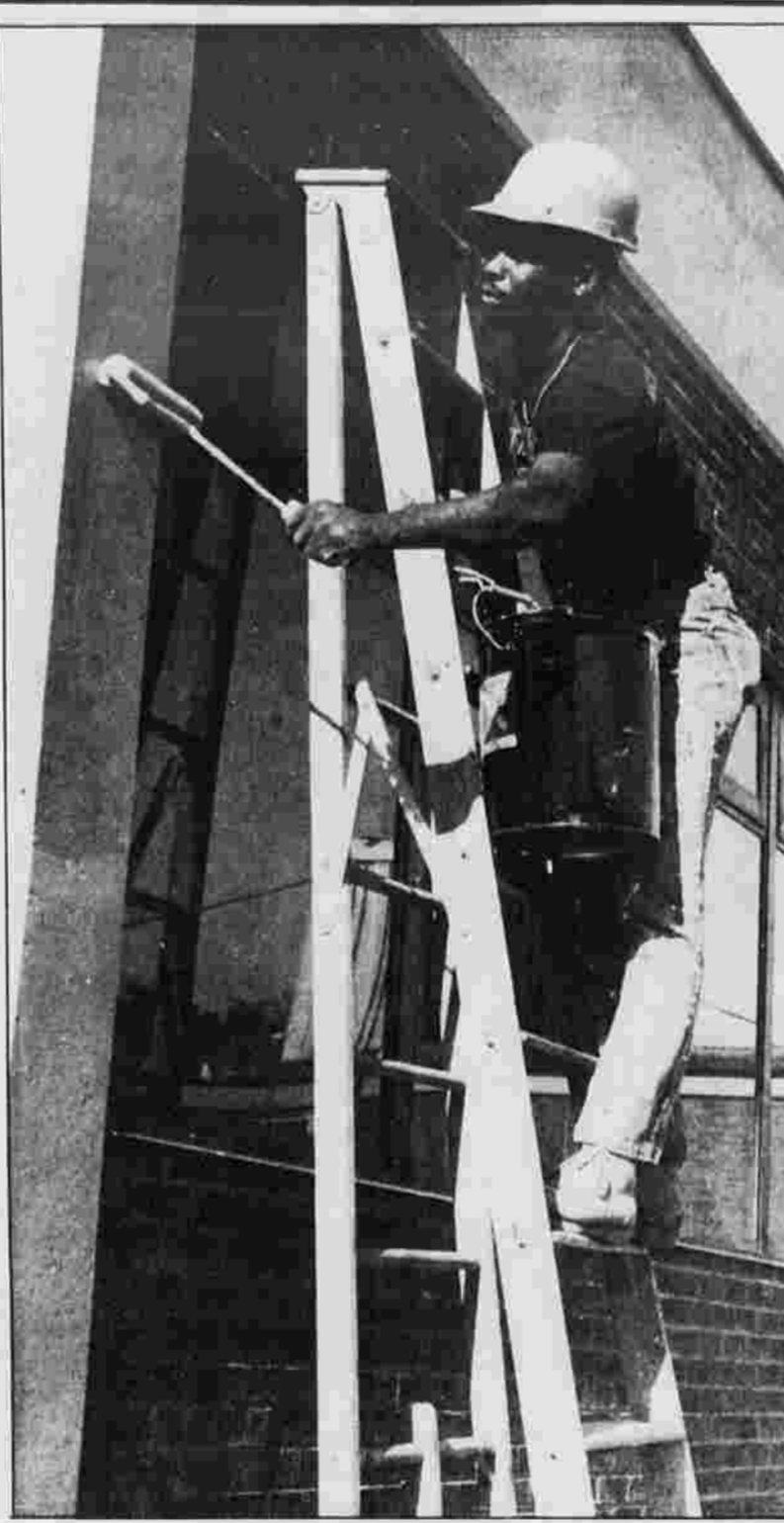
SPRUCE UP — Courtney Douglas of Bloomfield paints the side of the sewage treatment plant off Olcott Street Tuesday. The town is in the process of expanding the plant.
